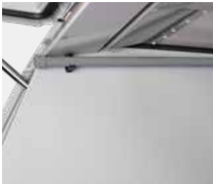
Snow bin wash system
