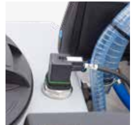
Fill level sensor in the tank
